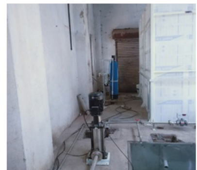
RO plant facility for IPX1 to IP X9K
